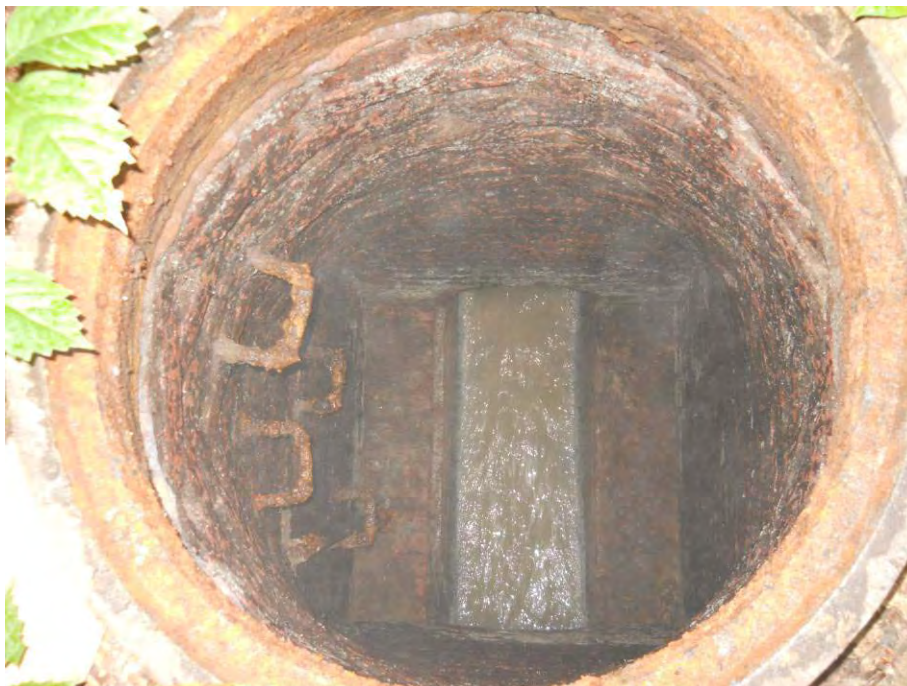
Photo – View of Sanitary Manhole M-9763 with corroded frame and steps
