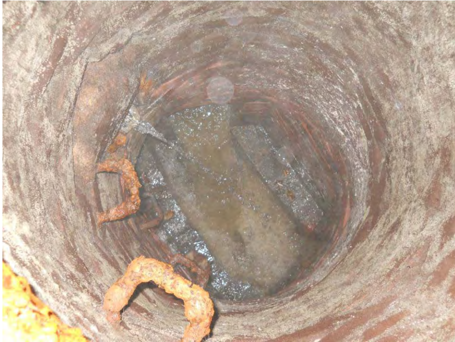
Photo – View of Sanitary Manhole M-10363 with 6-inch connection
