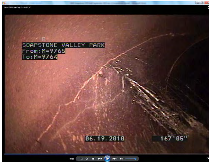
Photo – Example of crown of pipe with multiple cracks (Rotated View)
